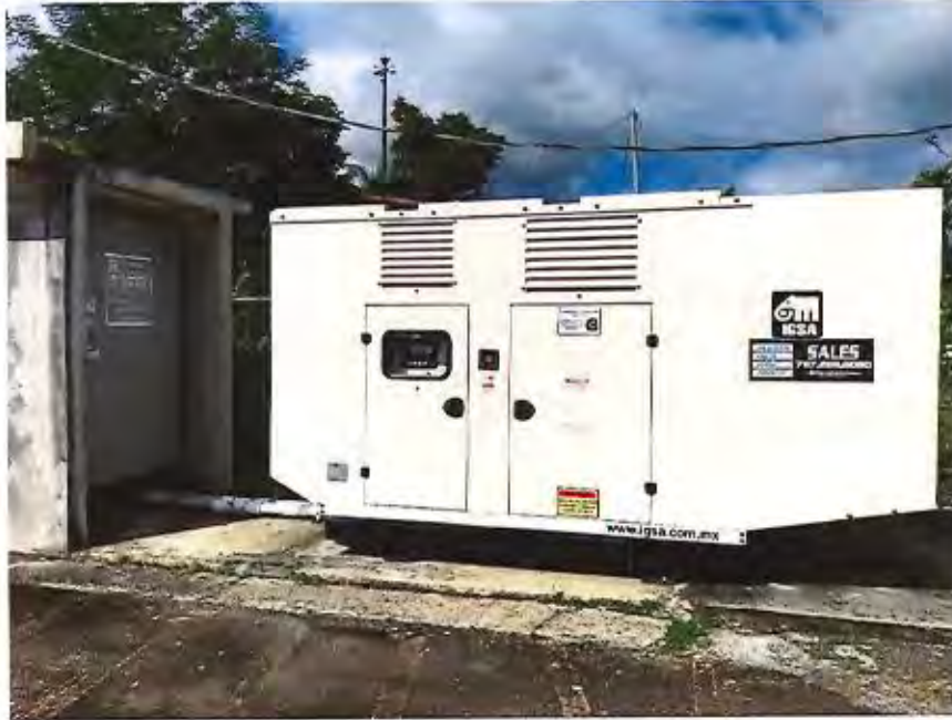
Figure 9: 250 KW Cummins Emergency Generator with self-contained diesel tank – Office of Secretary for Infrastructure, Beautification and Conservation
