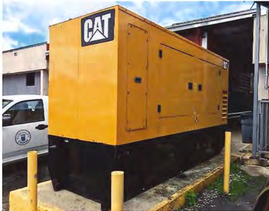
Figure 6: Emergency Generator with self-contained diesel storage tank – Building Conservation Department
