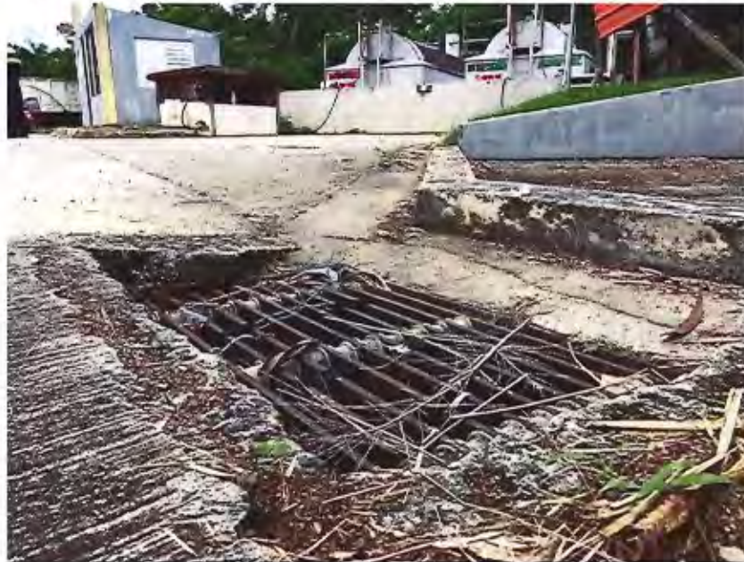
Figure 4: Storm Sewer near to the two (2) 10,000 gallons AST'S
