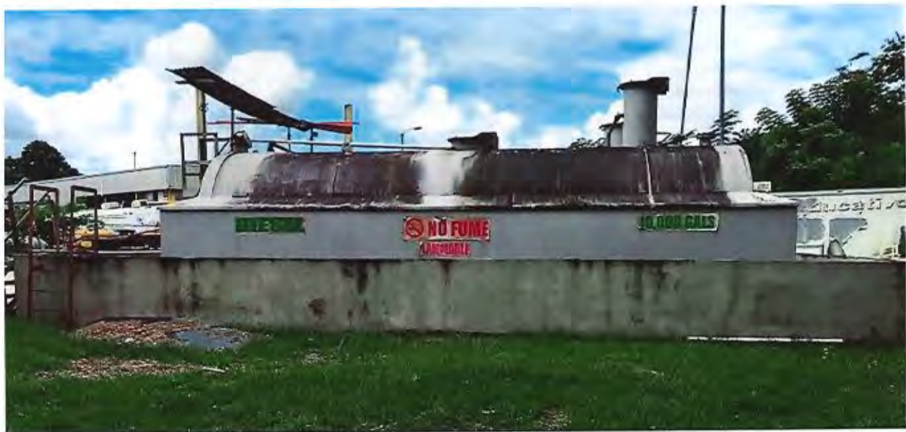
Figure 2: 10,000 Gallons diesel/gasoline aboveground store tanks (side view)
