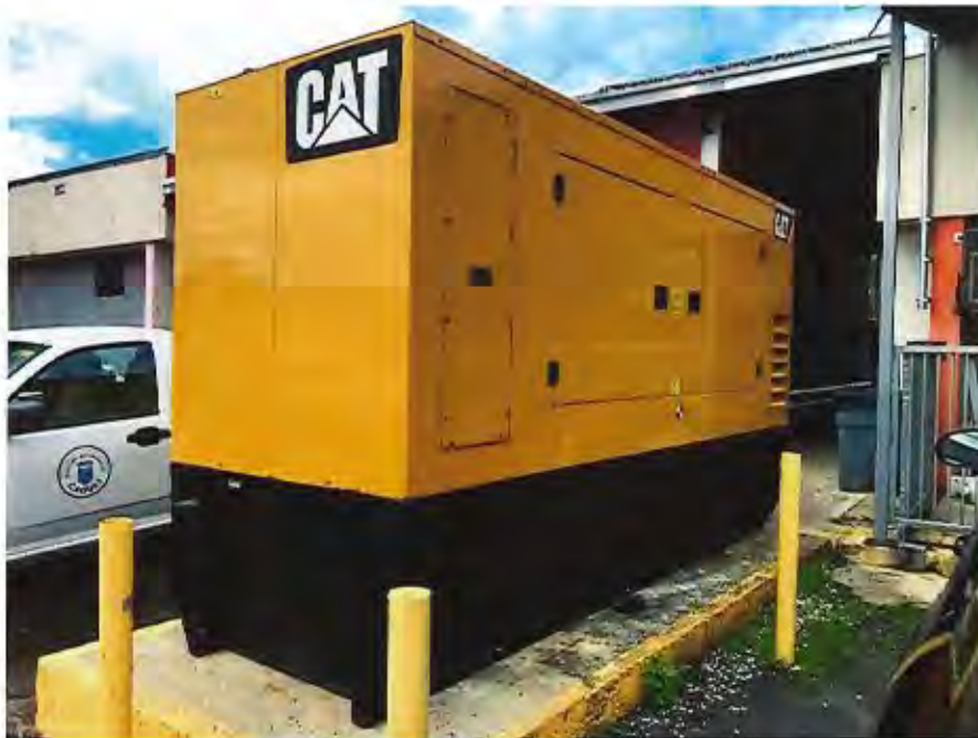
Figure 8: 200 KW Caterpillar Emergency Generator with self-contained diesel tank – Building Conservation Department
