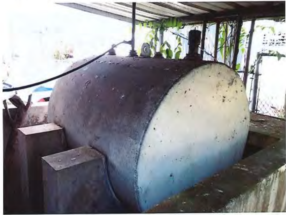
Figure 5: ~280 gallons AST near the wastewater treatment plant and its containment area
