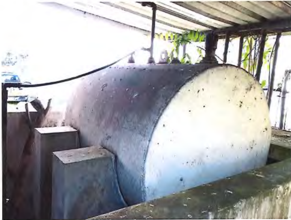
Figures 5 - 6: ~280 gallons Diesel Aboveground Storage Tank
