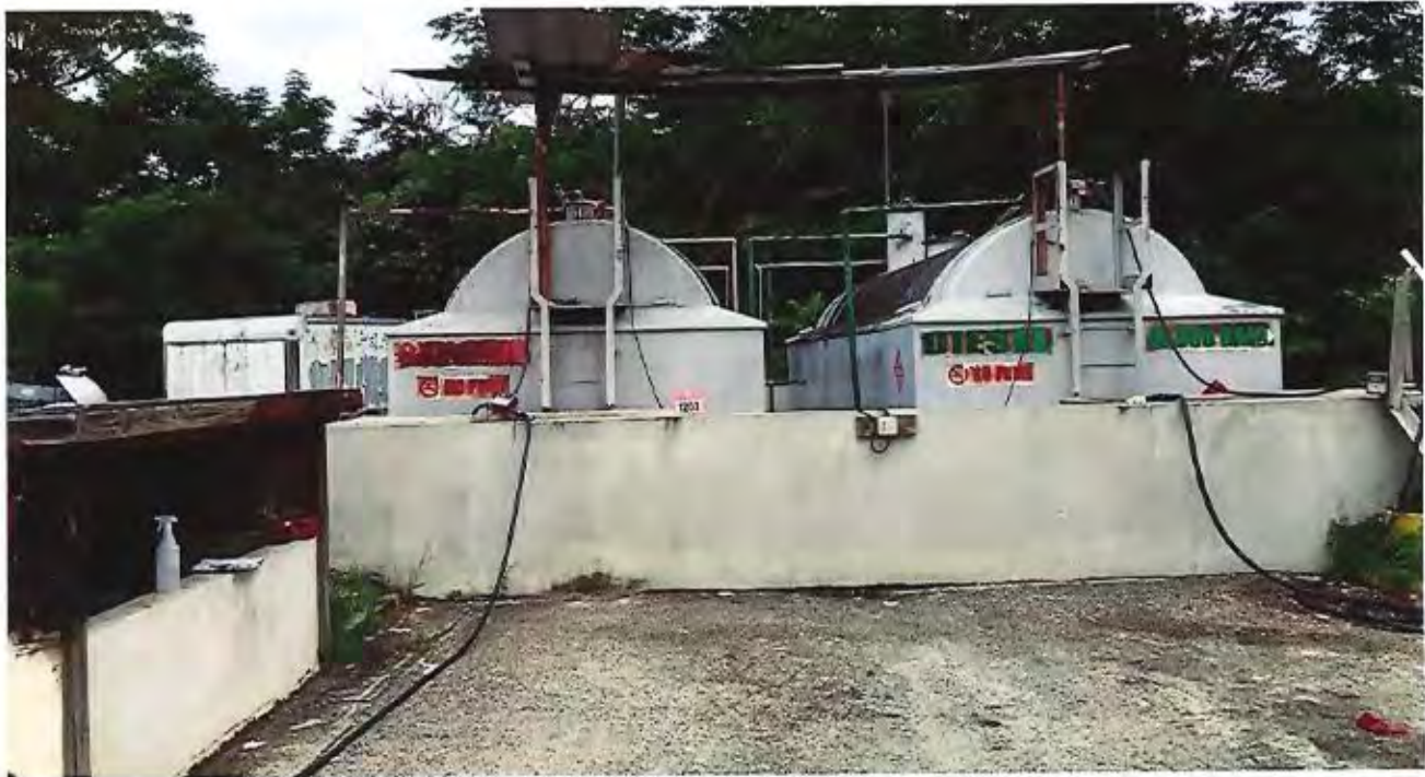
Figure 1: 10,000 Gallons diesel/gasoline aboveground store tanks (front view)
