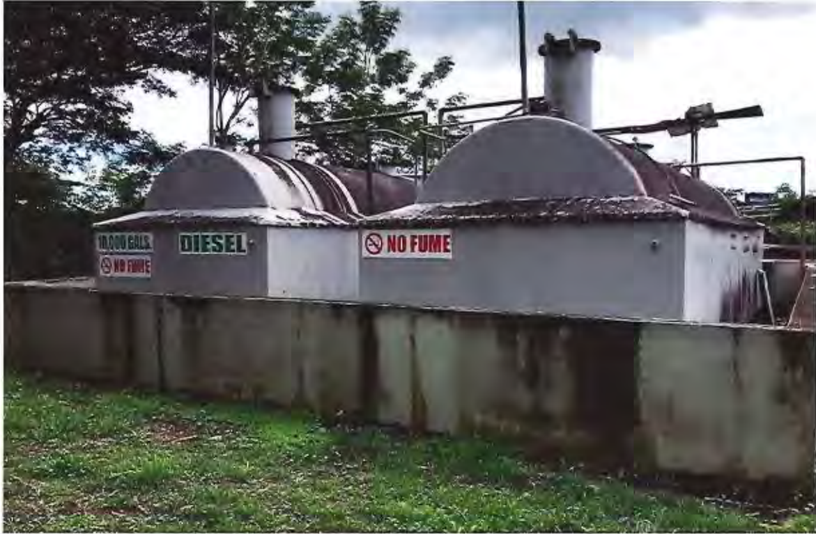
Figure 3: 10,000 Gallons gasoline/diesel aboveground store tank (rear view)
