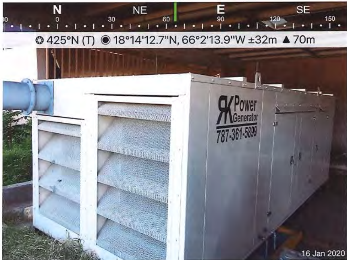
Figure 3: Self-contained emergency generator Perkins with integrated diesel tank of 250 gallons approximately.
