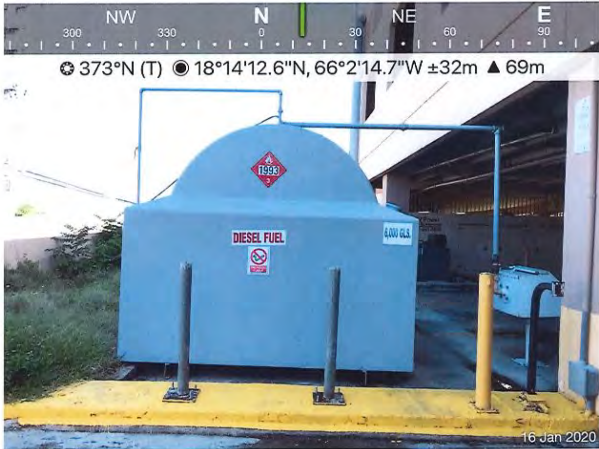
Figure 1: 6,000 Gallons diesel aboveground store tank (side view)
