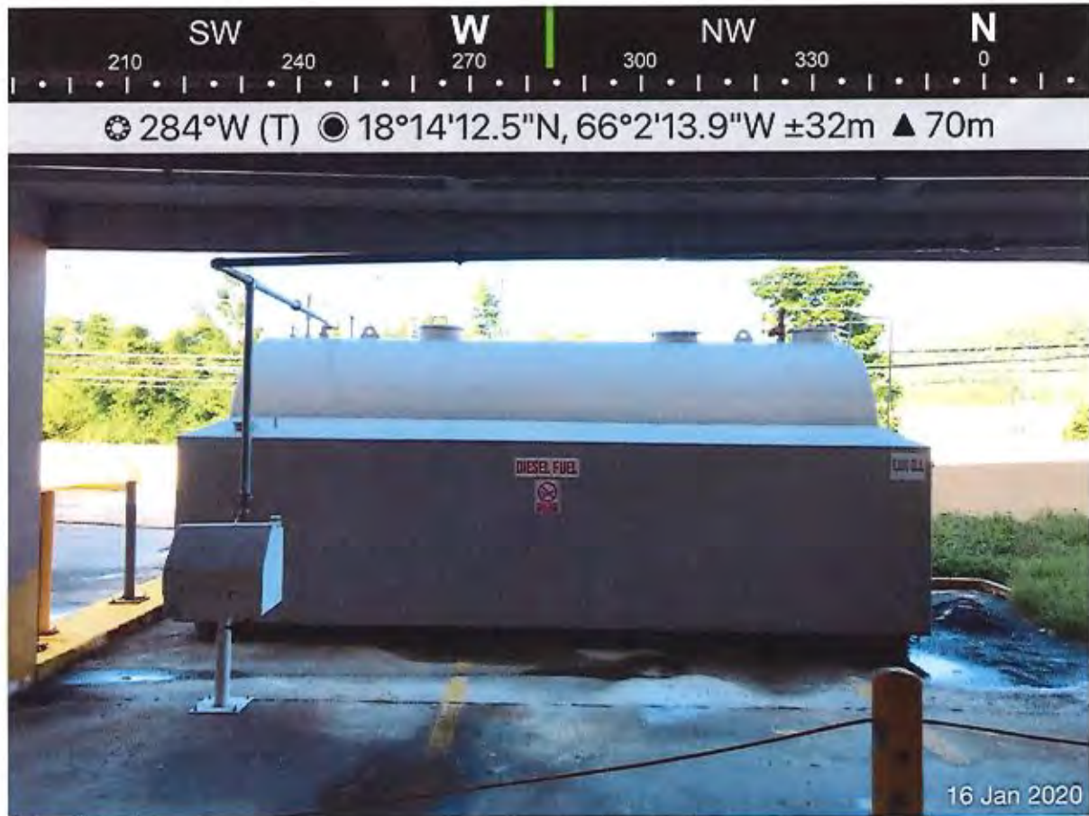
Figure 2: 6,000 Gallons diesel aboveground store tank (front view)
